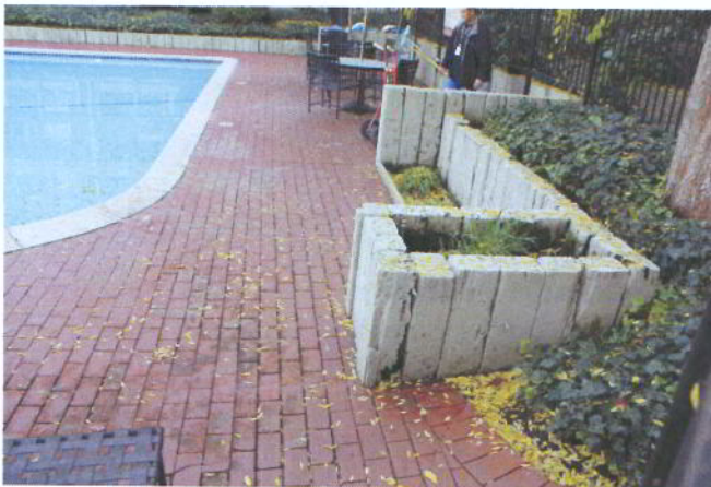
Photo 17 - Failing retaining and planters at pool.
