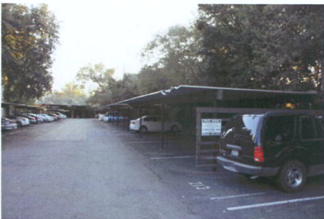
Photo 3 - Carports in poor repair.
