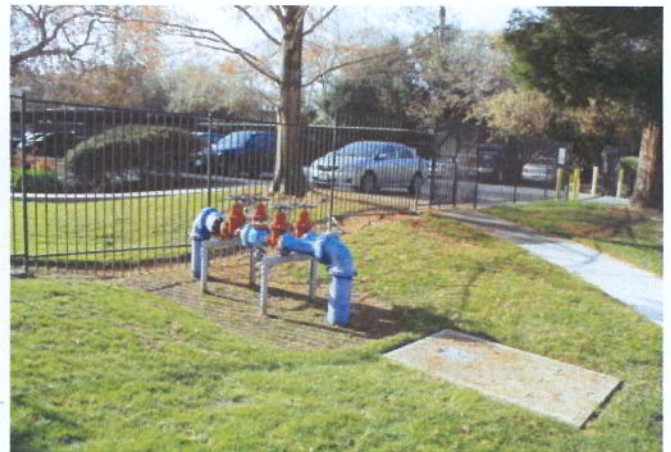
Photo 2 - Backflow device at entry.
