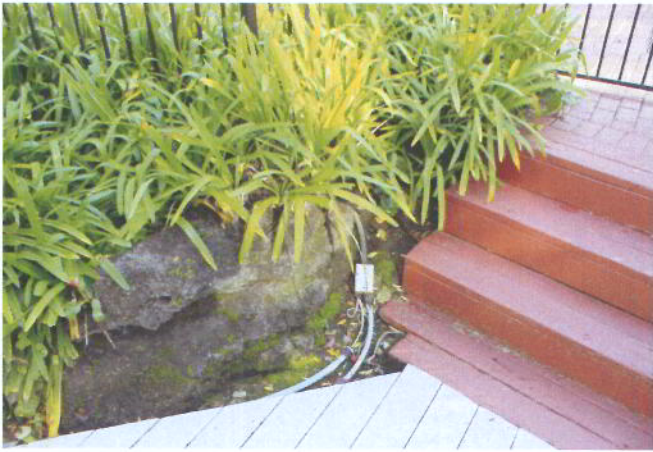
Photo 19 - Conduit with exposed wiring.
